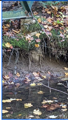
Erosion threatens the foundations of Case Bridge in the Aurora Sanctuary. Photo: B. Twaddell
