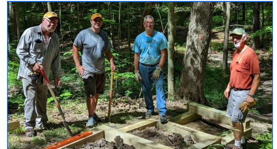
Keith Kohnke, Jim Tolan, Matt Valencic and Rob Swaney begin laying timbers for the new landscape stairway.
