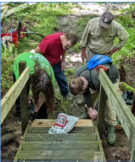
Hal Goodwin & Rick Deininger look on as Henry & Gus Burkhardt secure new steps to the damaged stairway.
