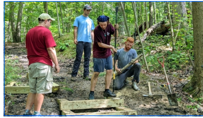
Jim Tolan, Neil Robertson, Aiden Stephens and Collin Himes from Hiram College position timbers.
