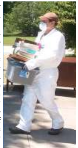
A member of the Hiram work crew, in protective gear against the dust of the Ed Center's attic, brings a load of materials outside for examination.
